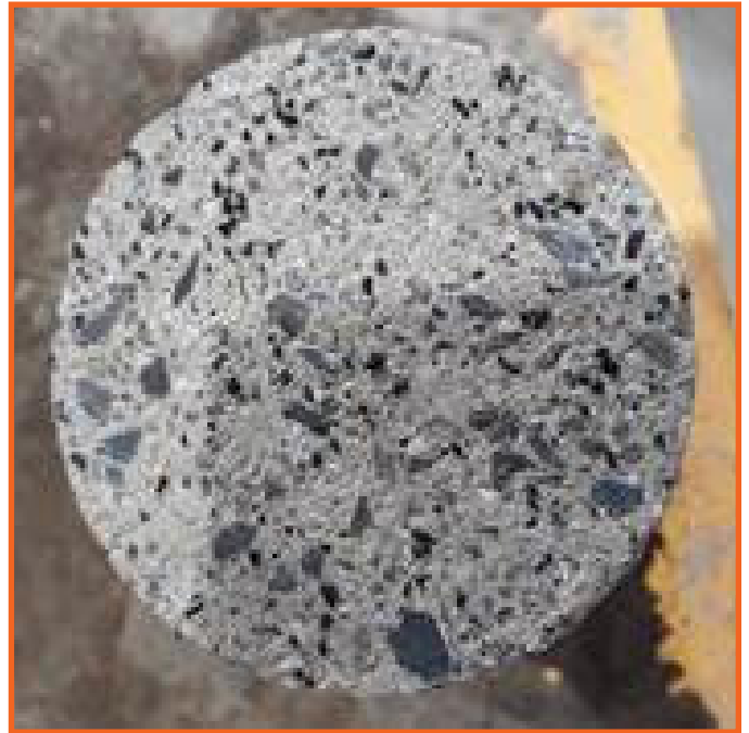
Concrete cylinder from pavement with recycled plastic and rubber fines
