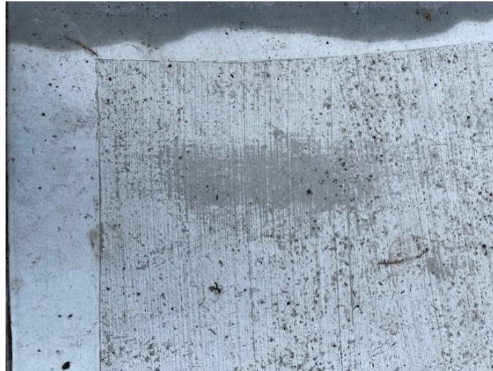
Fig. 6.18: Dusting on FBA concrete (after two months).
